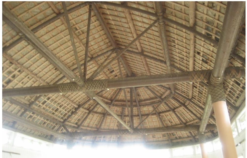
Roofing of the Tonga National Cultural Centre (interior) use coconut husk (kafa) for the lalava instead of nail.
